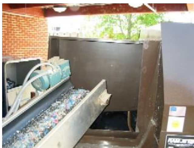
Sterile-Harmless end product discharging into compactor
